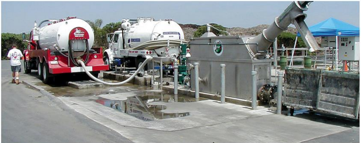
Proposed Septage Receiving Facility
