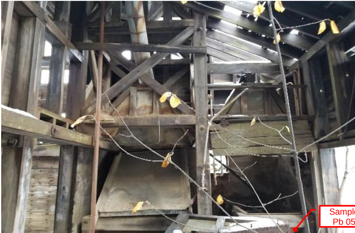
Photograph 13: Sand House – Interior 1st Floor Hopper. Orange Paint Chips (Lead, 25.4 mg/Kg, Both Entrances)
