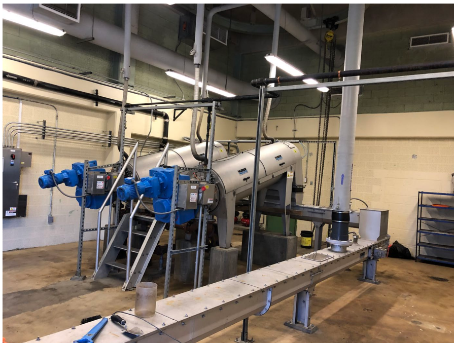
Existing Dual Sludge Dewater Huber Press System at WWTP
