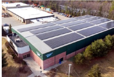
City of Nashua Transit Garage, Fire Dept, Ice Arena, Schools 1.6 MW (2019-20)
