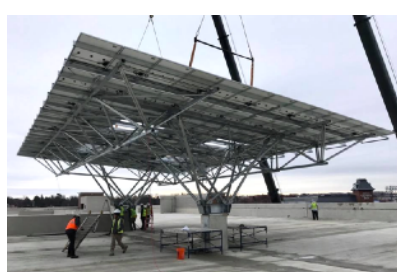
City of Manchester Langer Place Parking Garage (with SNHU); 1 MW RFP award (2019)
