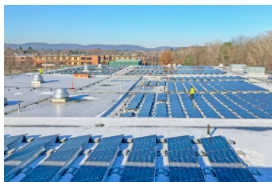
City of Keene Police Department, DPW, and WWTP 2.0 MW (2018, 2020)
