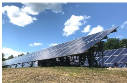
Town of Hooksett Wastewater Treatment Plant, 786 kW (2020) (2018 WWTP shown)
