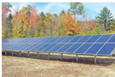
Town of Springfield Village District of Eastman (WWTP) 260 kW (2016)
