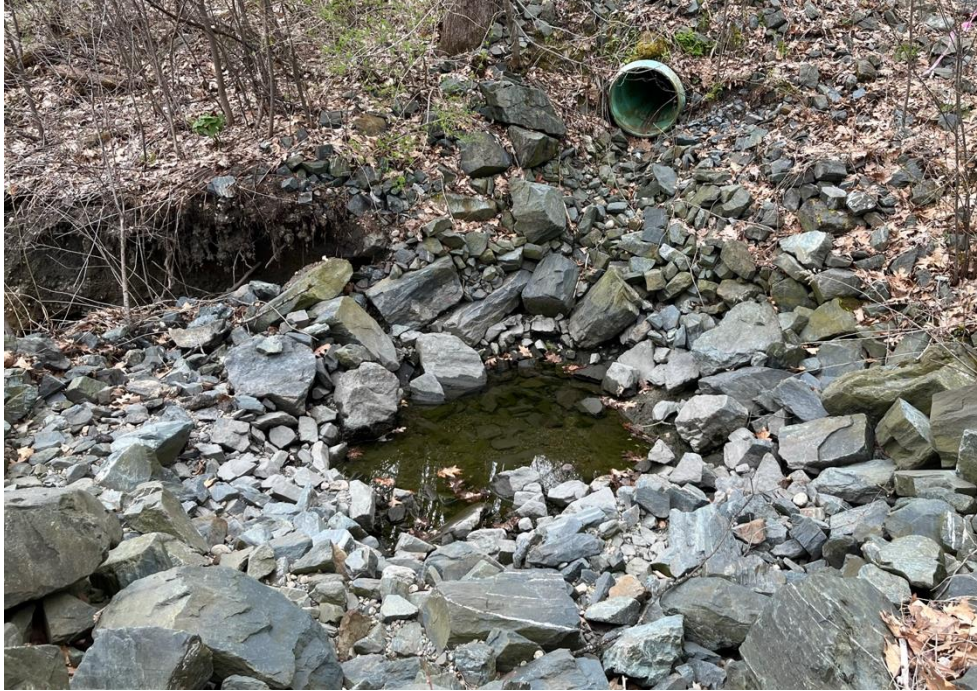
Image 1: Plunge Pool at Outlet of 24-inch Diameter Culvert (Outfall No. 1)
