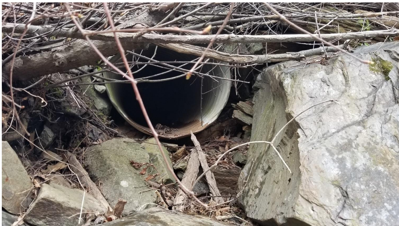
Photo 9. LS1 outfall to Mascoma River (end).
