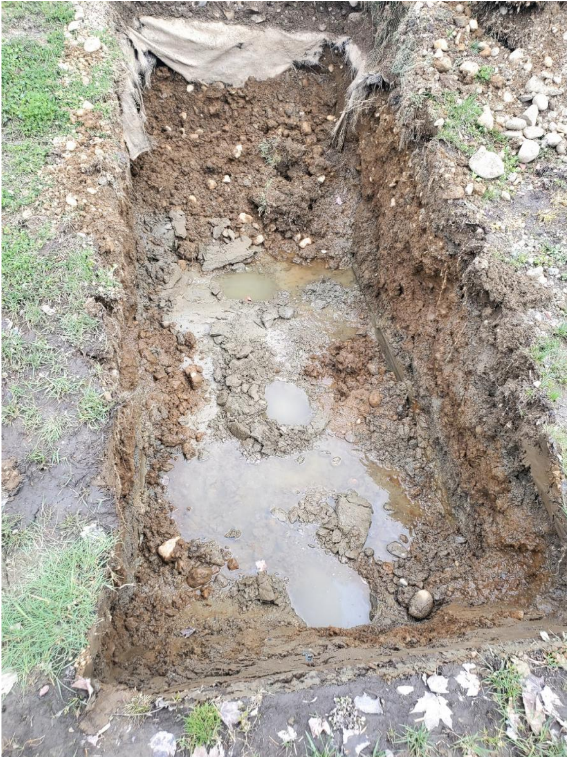
Water conditions after approximately 2.5 hours.
