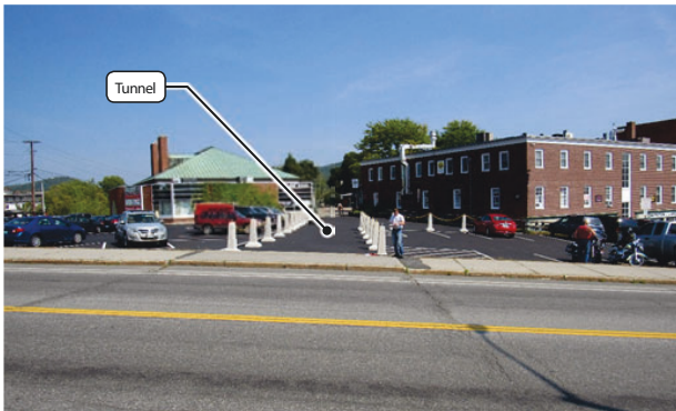
THE TUNNEL IS BARRICADED TO KEEP VEHICULAR TRAFFIC OFF THE SUPERSTRUCTURE
