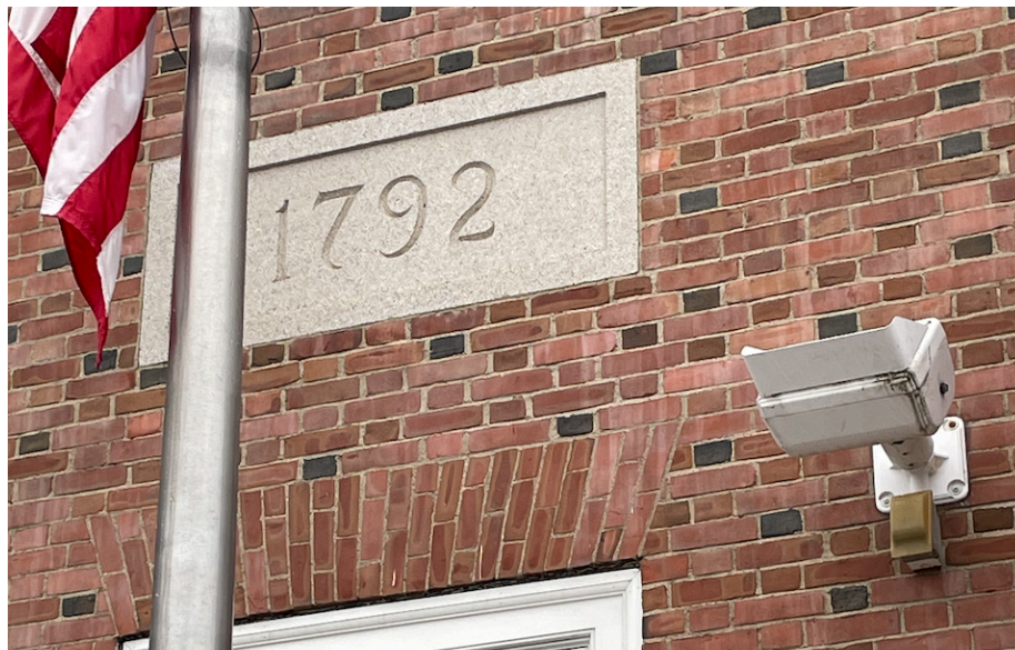
Existing Flag Floodlight
