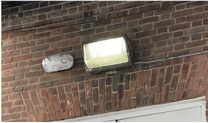
Existing Safety Floodlight
