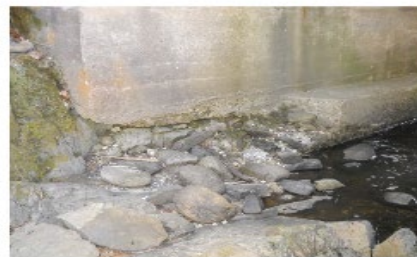
Abutment Concrete Spalling
