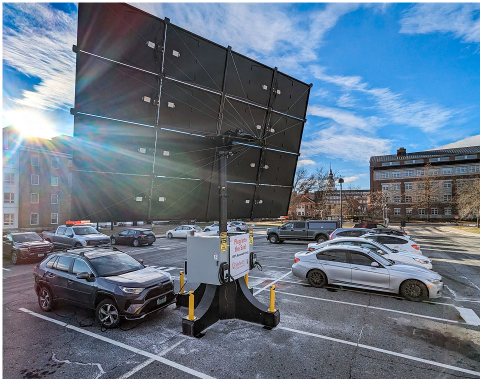
Solar EV Charger, Dartmouth College
