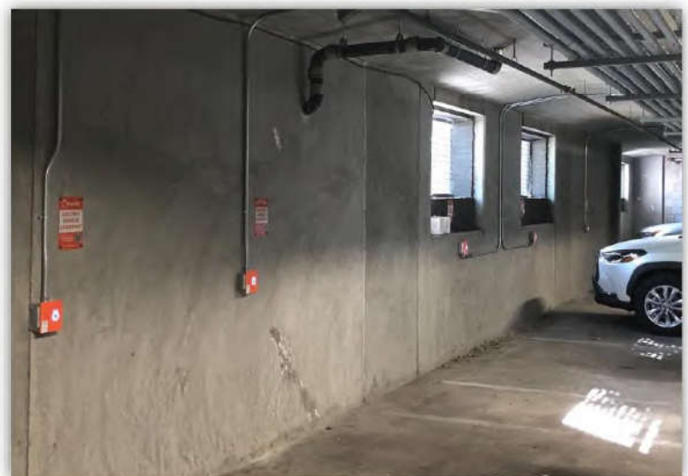
EV chargers installed through PCE "EV Ready" program
