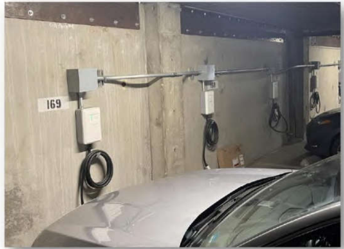
EV chargers installed through PCE "EV Ready" program
