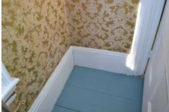
Left: Softwood floor of the room behind (west of) the front sitting room
