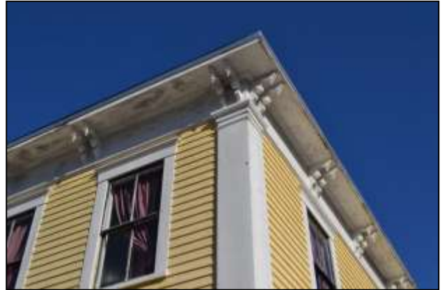
Cornice at south (right) elevation and elevation (left), showing the continuity of casings and cornice design on all elevations.
