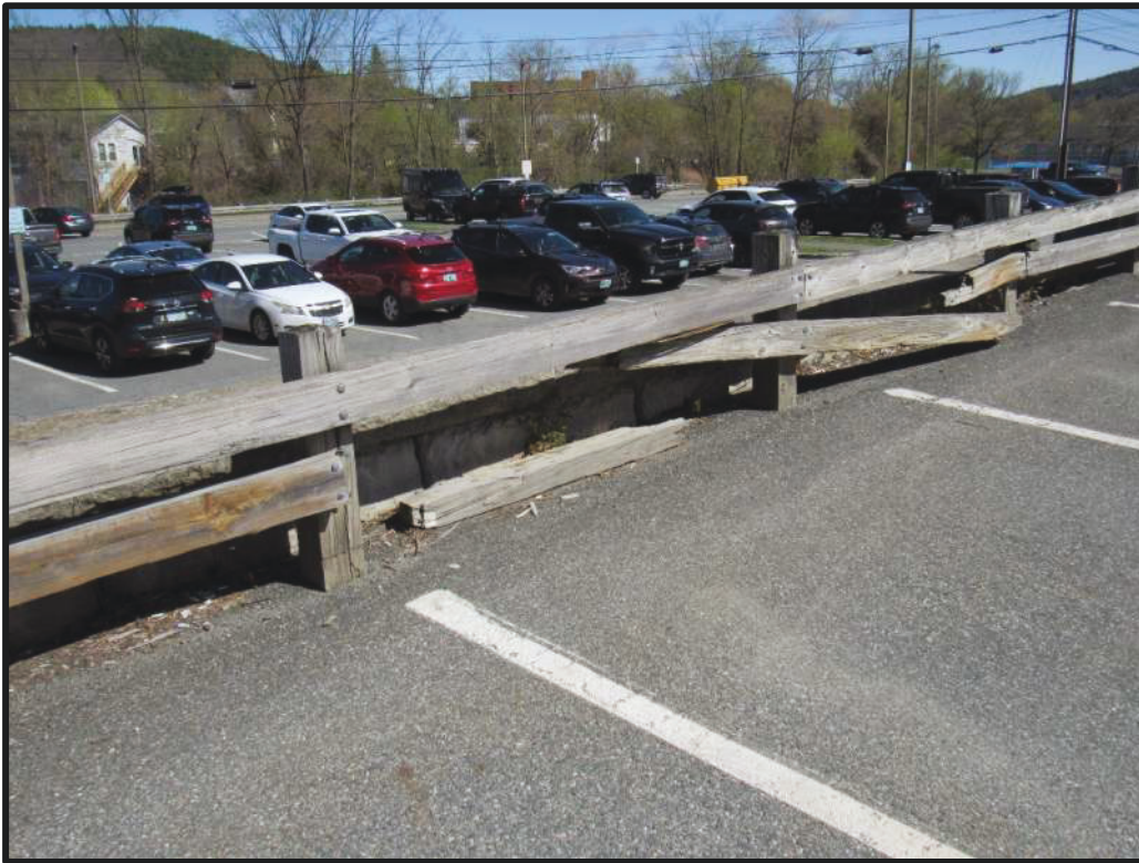
Photo 16 – Broken Railing Members in Guardrail Segment #1
