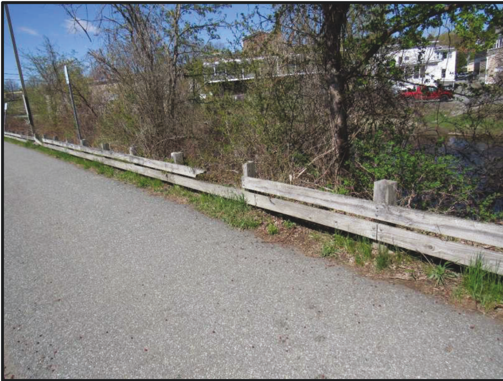
Photo 18 – Broken Railing Members in Guardrail Segment #2
