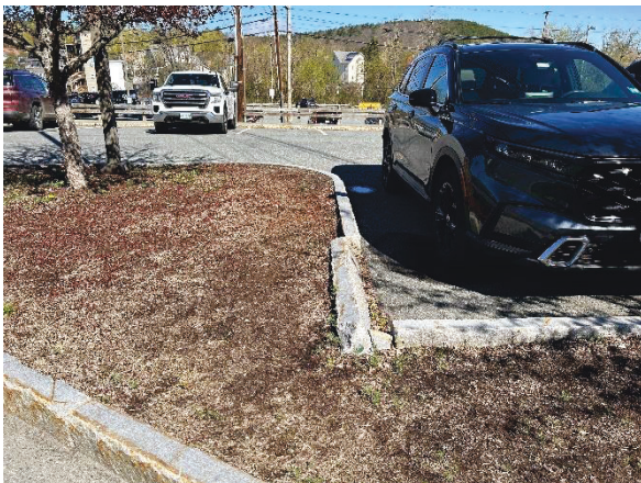
Image 9. Curb Condition (West view)
