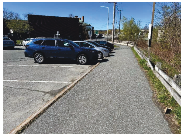
Image 4. Sidewalk Condition (Southwest View)
