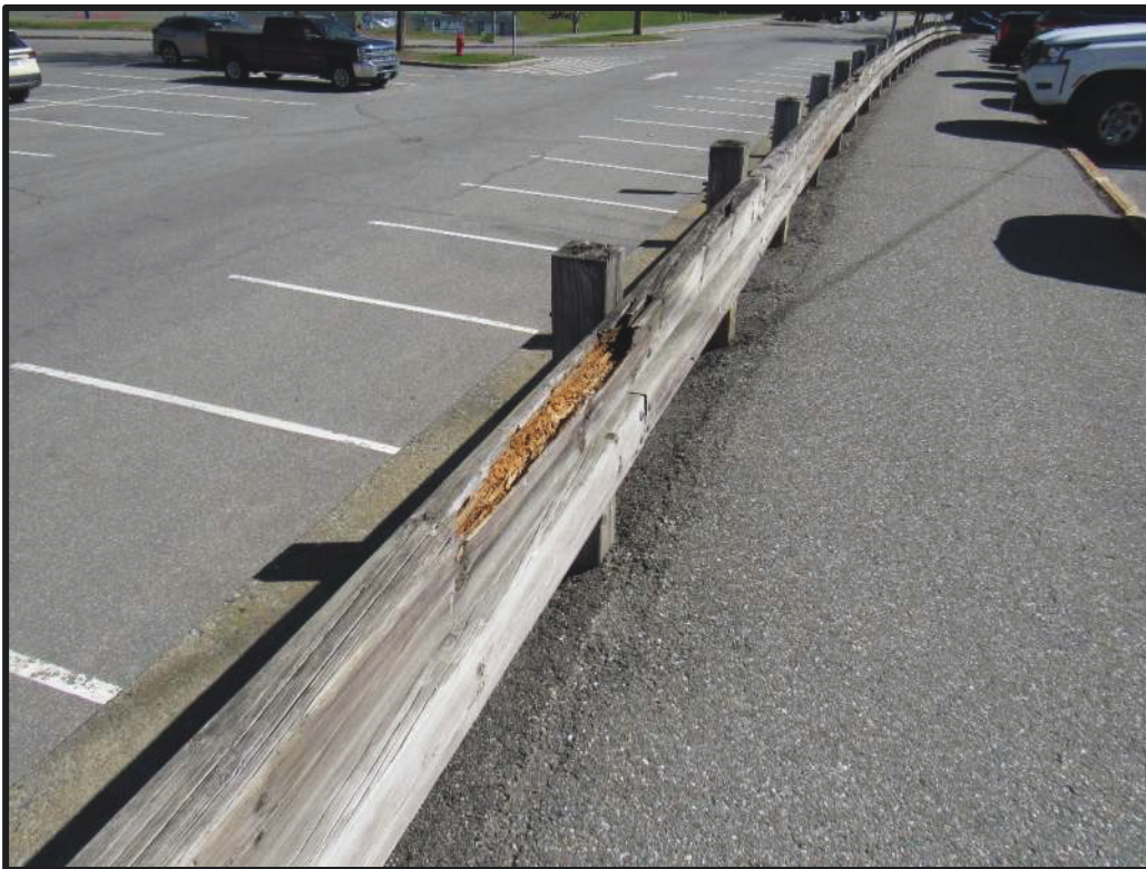
Photo 15 – Deteriorated Railing Members in Guardrail Segment #1
