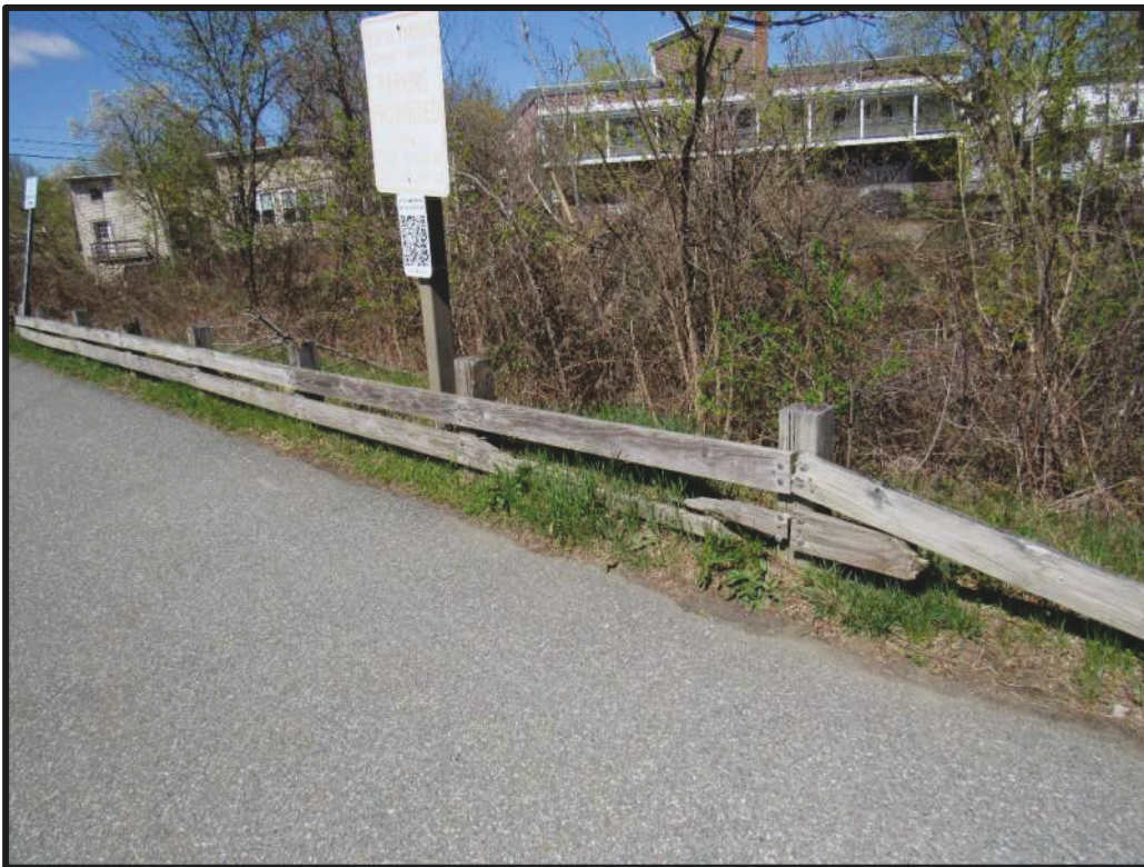
Photo 19 – Broken Railing Members in Guardrail Segment #2
