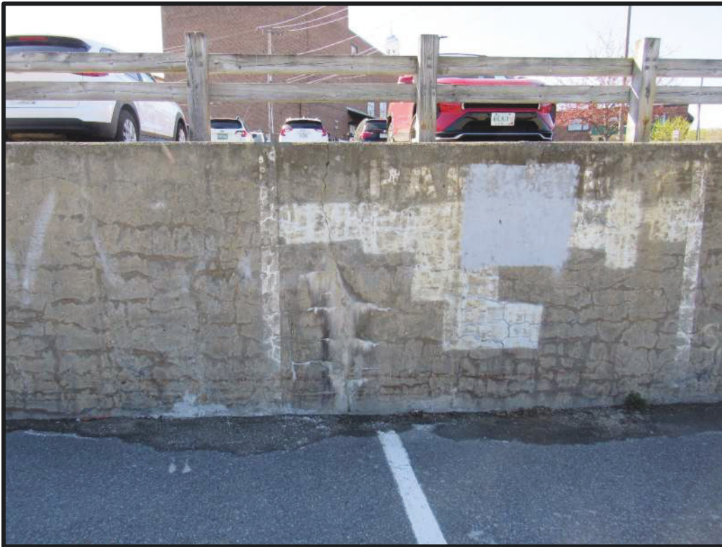
Photo 8 – Map Cracking and Efflorescence on Wall Segment #2
