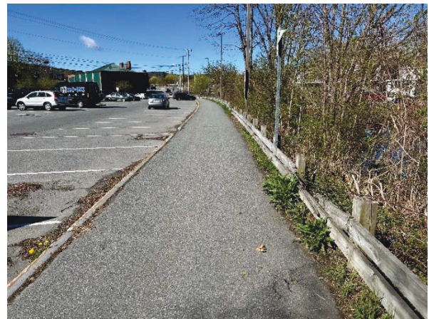
Image 2. Sidewalk Condition (Southwest View)
