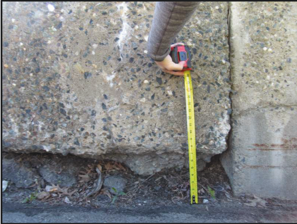
Photo 6 – Void Under Block in Wall Segment #1
