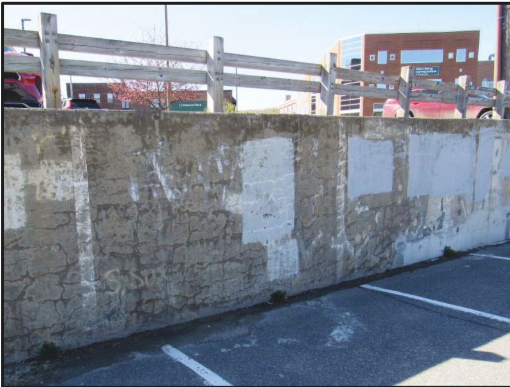
Photo 9 – Map Cracking and Efflorescence on Wall Segment #2
