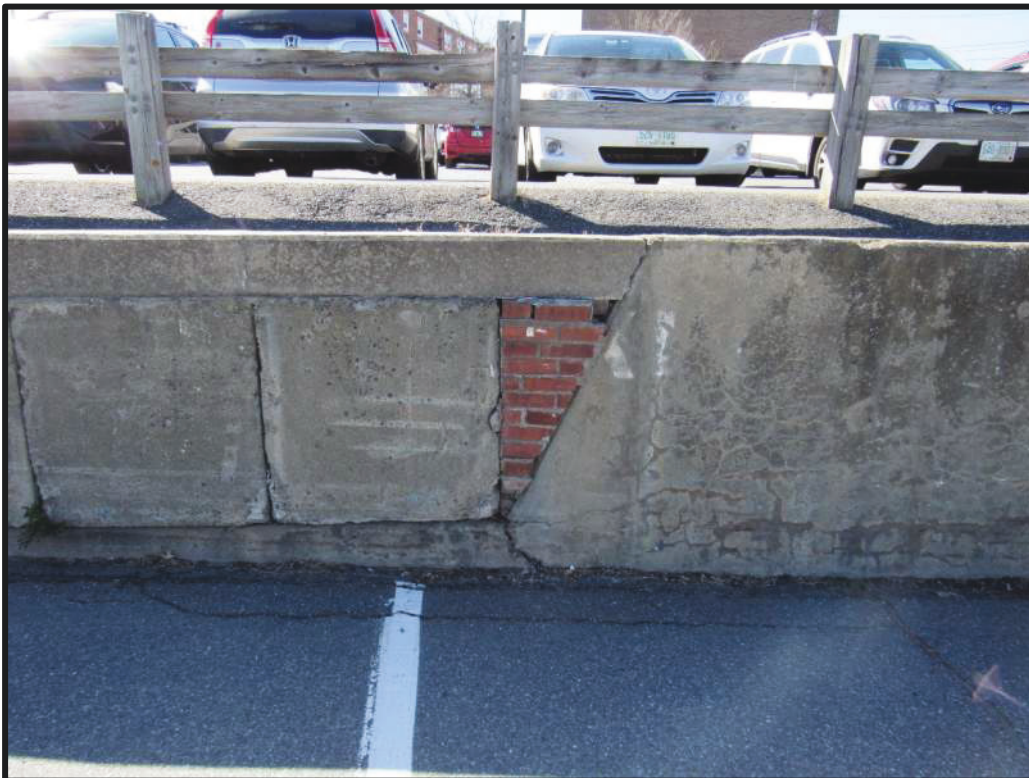
Photo 7 – Loose Bricks Between Wall Segment #1 and #2
