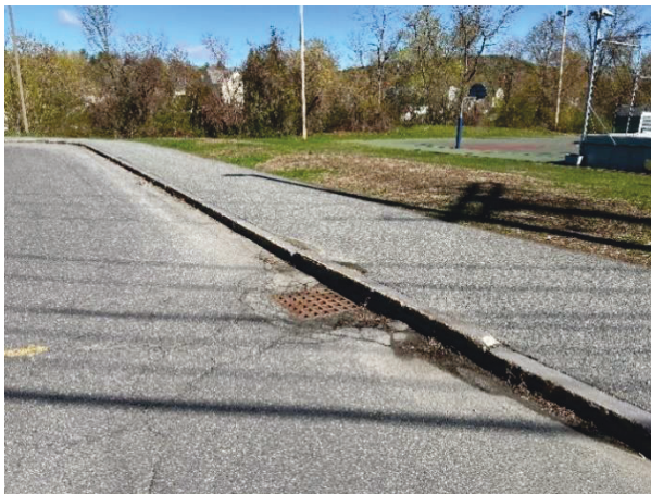
Image 1. Sidewalk Condition (Northwest view)
