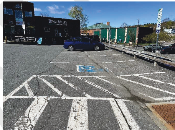
Image 10. Pavement Condition (South View)
