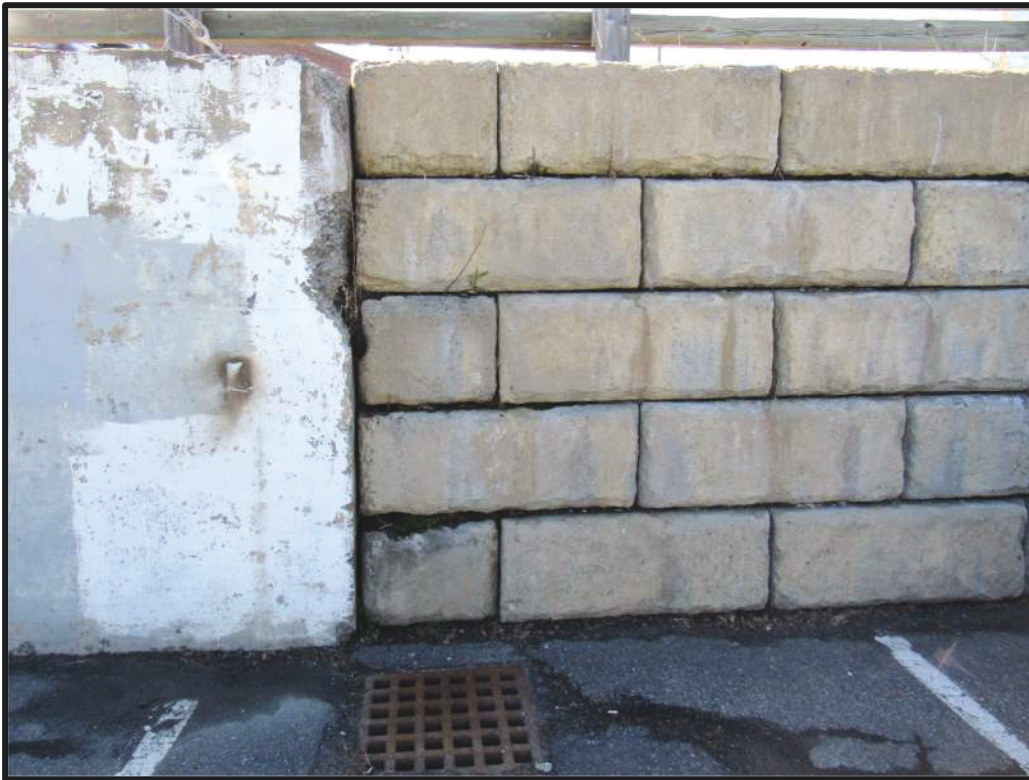
Photo 12 – Vegetation Growing Between Joints in Wall Segment #3
