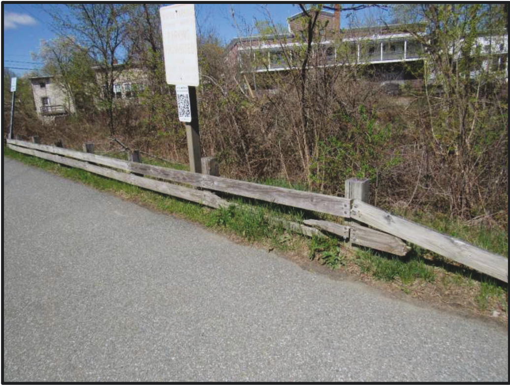
Photo 19 – Broken Railing Members in Guardrail Segment #2
