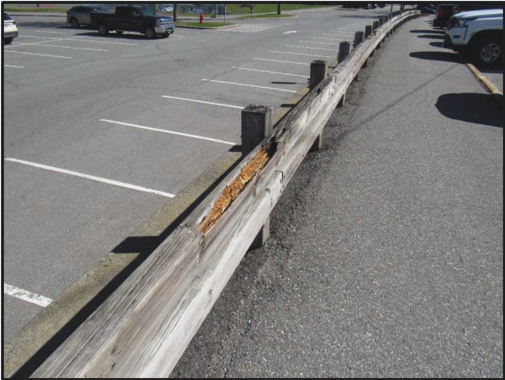
Photo 15 – Deteriorated Railing Members in Guardrail Segment #1
