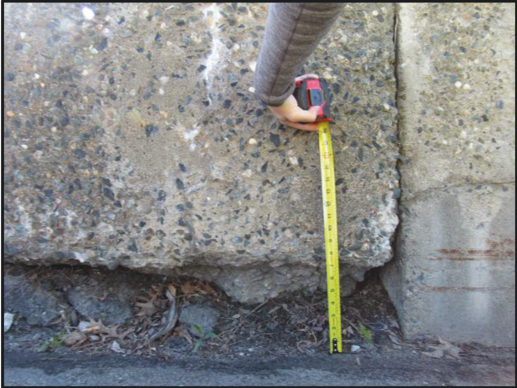
Photo 6 – Void Under Block in Wall Segment #1
