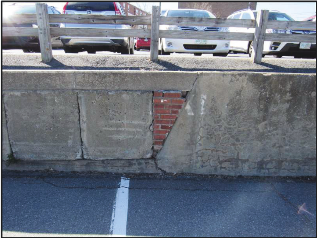
Photo 7 – Loose Bricks Between Wall Segment #1 and #2
