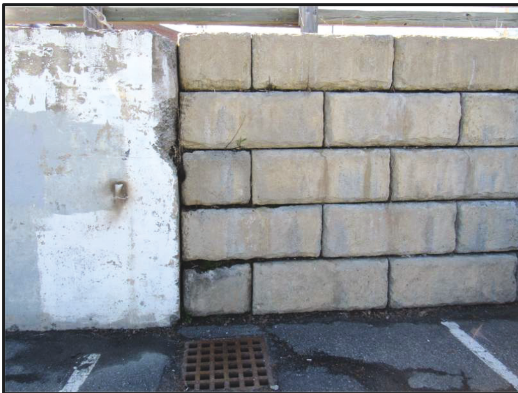
Photo 12 – Vegetation Growing Between Joints in Wall Segment #3
