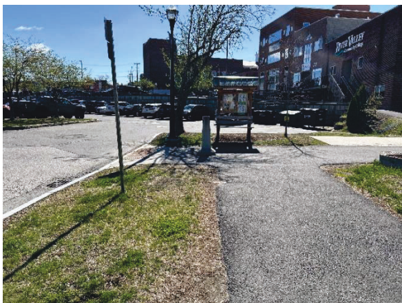
Image 5. Sidewalk Condition (Southeast view)
