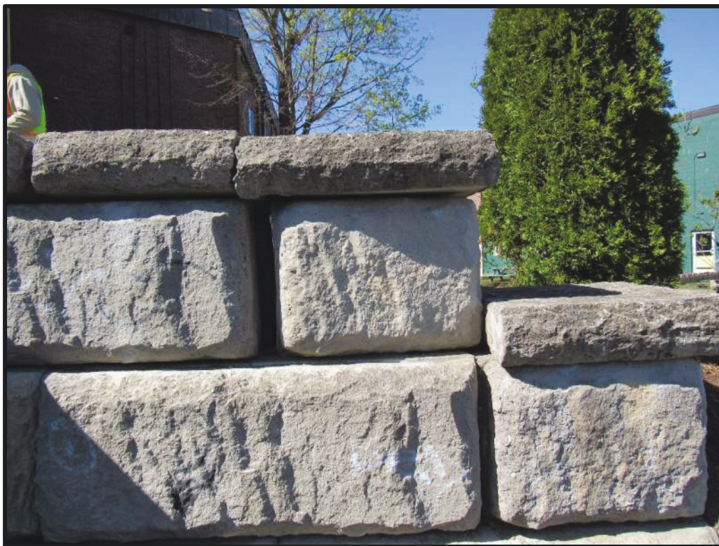
Photo 13 – Loose Block and Crack in Cap of Wall Segment #3 Return Wall
