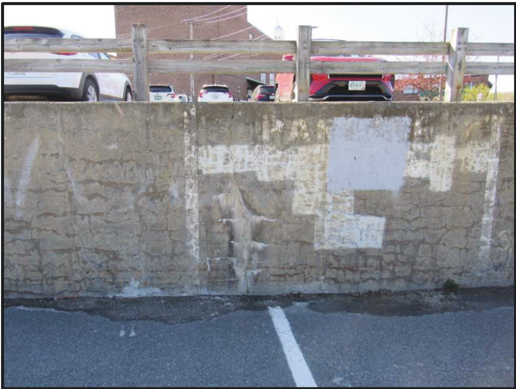
Photo 8 – Map Cracking and Efflorescence on Wall Segment #2
