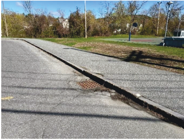
Image 1. Sidewalk Condition (Northwest view)
