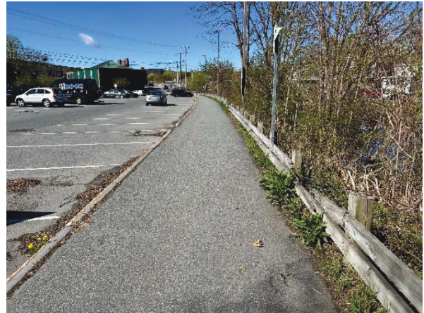
Image 2. Sidewalk Condition (Southwest View)
