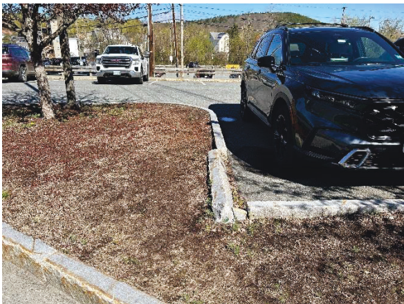
Image 9. Curb Condition (West view)
