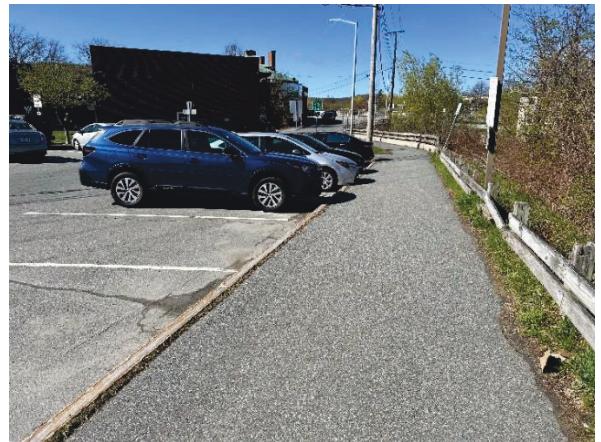
Image 4. Sidewalk Condition (Southwest View)
