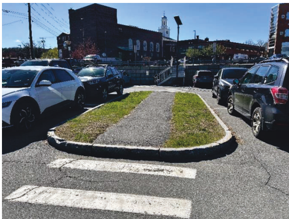
Image 3. Sidewalk Condition (Southeast View)
