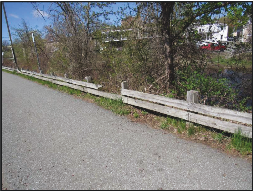
Photo 18 – Broken Railing Members in Guardrail Segment #2
