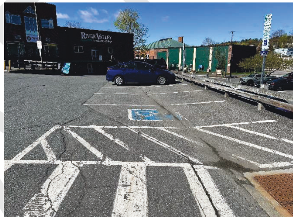
Image 10. Pavement Condition (South View)
