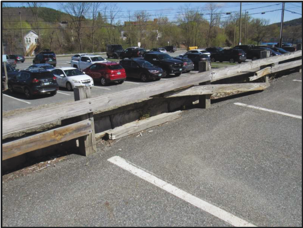
Photo 16 – Broken Railing Members in Guardrail Segment #1
