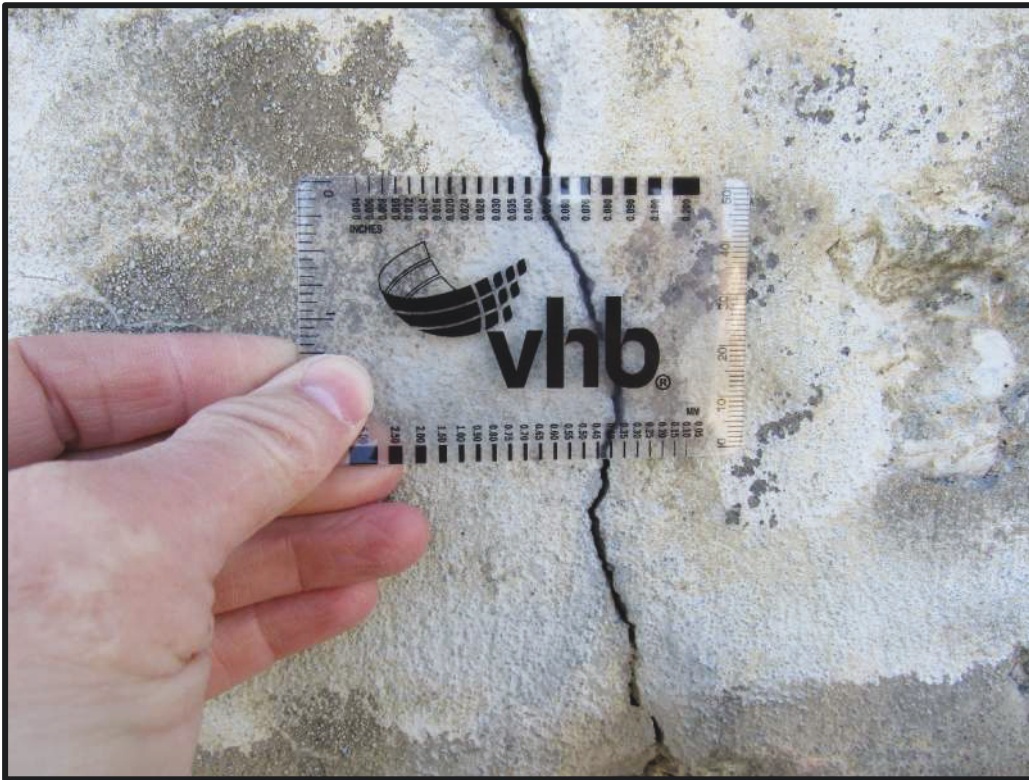
Photo 10 – 1/16 th Inch Wide Vertical Crack on Wall Segment #2
