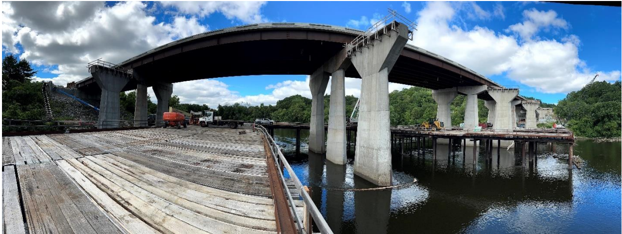
Photo 7: Upstream face of bridge, showing NH bank to the left and VT bank to the right (7/18/2025)
