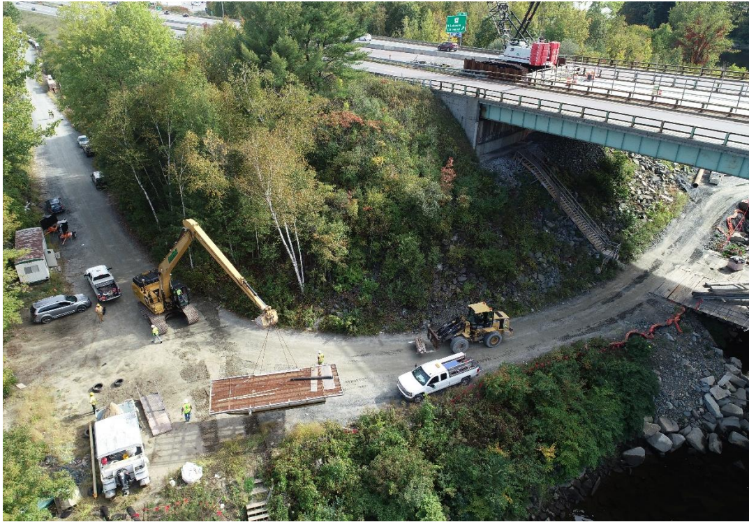
Photo 5: Facing New Hampshire side, northeast bridge quadrant, impact areas D, E and F (10/03/2022)
