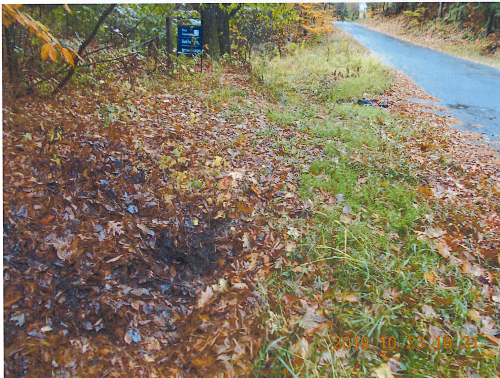
Photograph No. 2 (dated 10/23/19): View to the southwest showing the inlet end of the existing culvert under the woods road that is buried with accumulated sediment.
