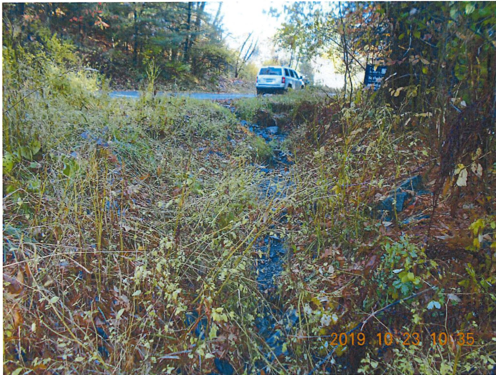
Photograph No. 9 (dated 10/23/19): View to the north showing the eroded ditch downgradient of the culvert under the woods road.
