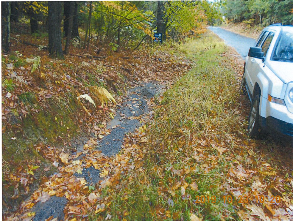
Photograph No. 1 (dated 10/23/19): View to the southwest showing the accumulated sediment in the road ditch up-gradient of the existing woods road and culvert.
