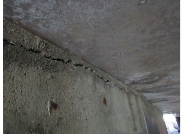
Figure 2.1 – cracking at top of abutment
