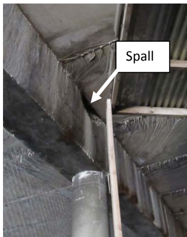
Figure 2.2 – Pier cap spall
