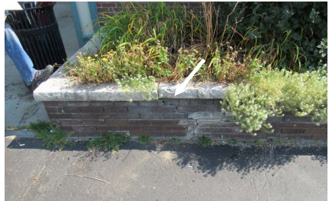
Figure 2.6 – Settlement crack at planter
